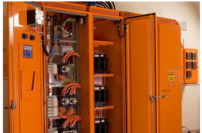
Figure 3: Berri Estate's Power Factor Correction Unit
