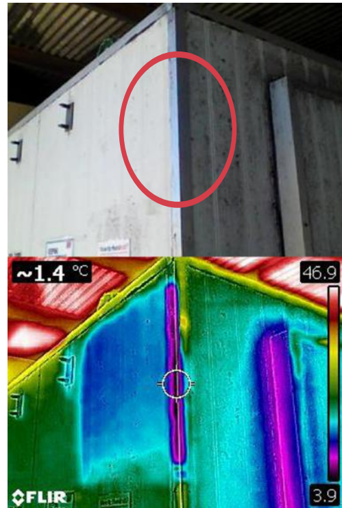
Hidden damage inside cool room
